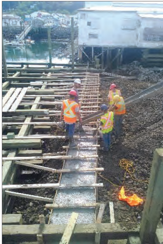
The wall between the wharf and the building creates the end of the foundation wall facing the harbour. It forms an integrated retaining wall that holds the building and prevents any storm surge from pounding in under the building and washing out the aggregate.
