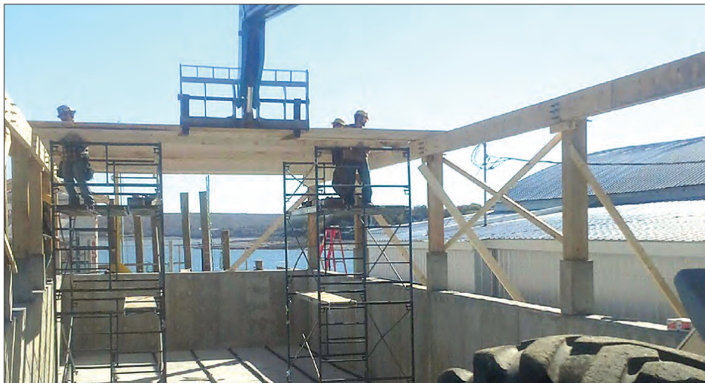
Rural Roots Engineering & Design of Masstown, N.S., in association with Brent Thornhill, owner and senior engineer with North Shore Engineering Inc. in Tatamagouche, designed and is overseeing construction of the project while M.R. Poole Excavating in Hampton, N.S. was the contractor.
